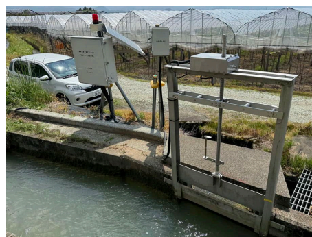
写真-1 遠隔制御対象の緊急放流ゲート Remotely controlled emergency release gate
